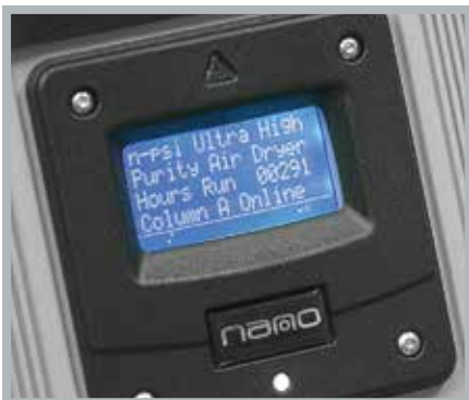
PLC controller with clear text display
